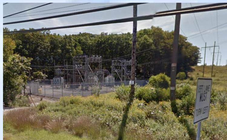
Substation from Google Map
