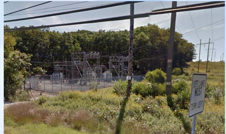
Substation from Google Map
